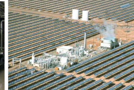
Solar thermal power generation
